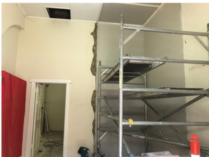
Left to right: New floor joists and beams in front of the arch—getting ready for more compactus storage. The photocopier area.
